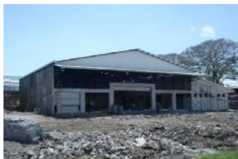
Center for the Recuperating of Recyclable Materials in Hatillo in its construction phase. April, 2010
